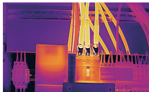
Electric Routine Inspection
