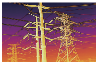
Electric Routine Inspection
